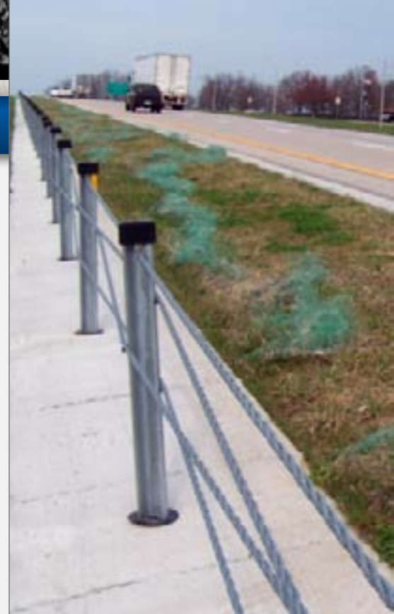
Cable Barrier Project with ECB Issues
